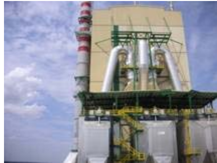
Figure S7. Kraft Mill Recovery Furnace
