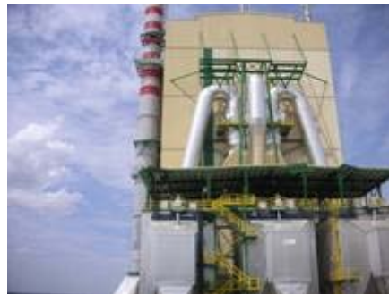
Figure S7. Kraft Mill Recovery Furnace
