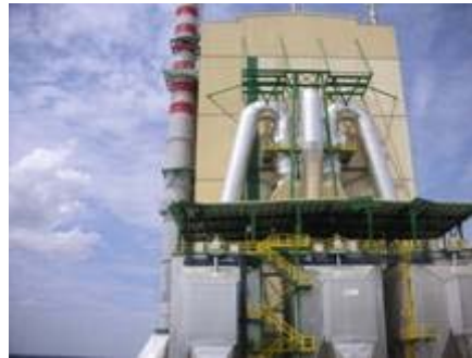
Figure S7. Kraft Mill Recovery Furnace
